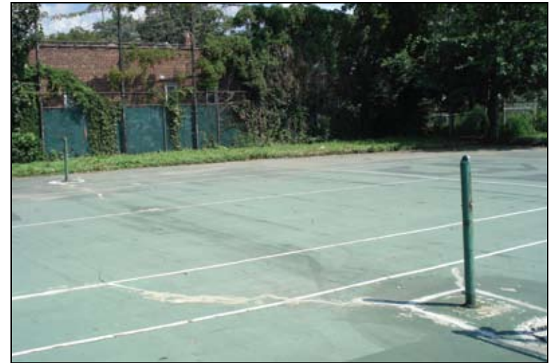
Flushing Fields, Queens: This tennis court is missing a net and is in desperate need of maintenance, with cracks and worn out areas in need of attention.
