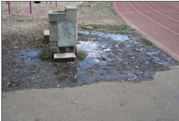
Leaks were a common problem among drinking fountains in McCarren Park.
