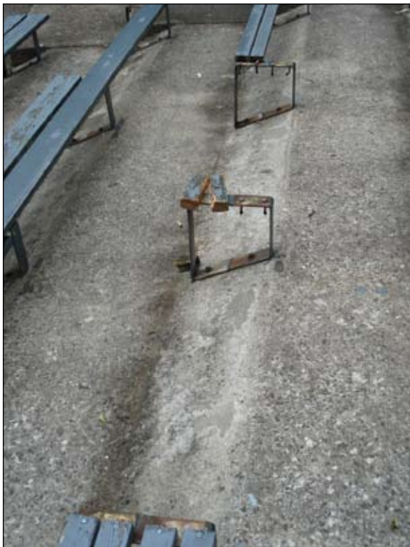
Many sitting areas are in need of repair.
