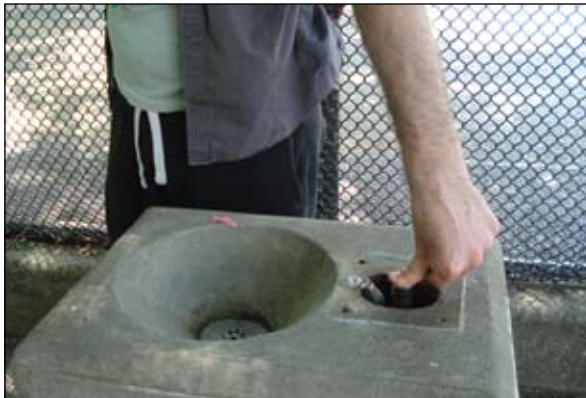
A number of drinking fountains lacked sufficient water pressure.
