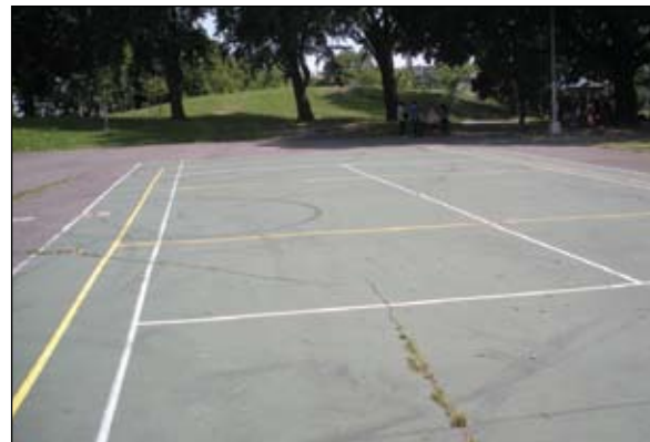
Severe cracks and a missing net impede play at this tennis court.
