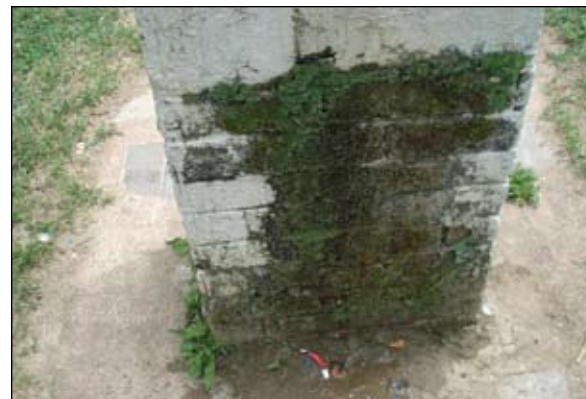
Mold grows around the base of this drinking fountain.
