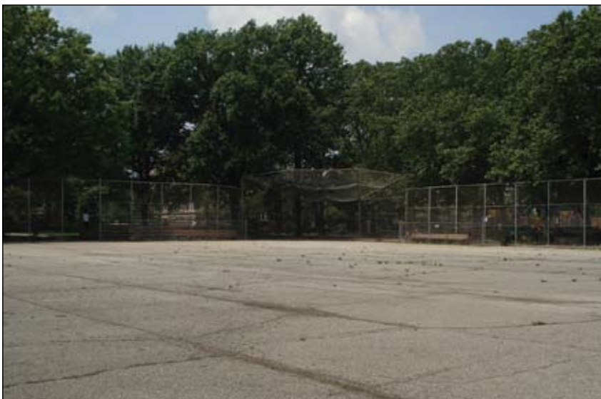
This asphalt baseball field is covered in cracks, posing trip hazards to users.
