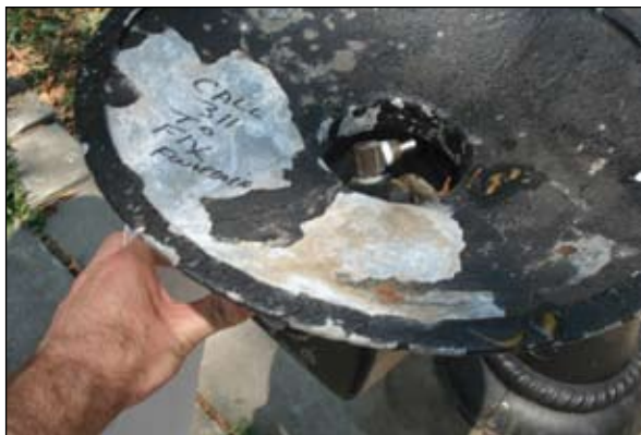
This water fountain is structurally damaged.
