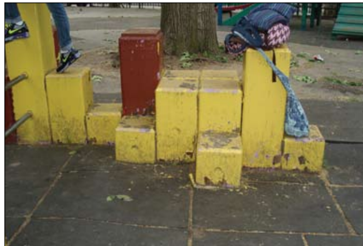
Playground equipment is worn, and safety surfacing is uneven.
