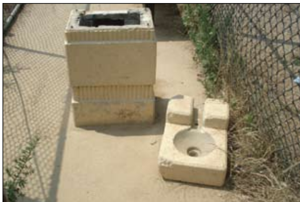
Multiple fountains at Coney Island Boat Basin were disconnected and unusable.
