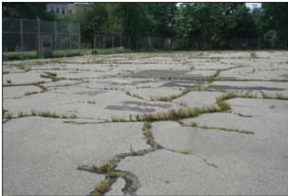
Large cracks run across the surface of this asphalt baseball field.
