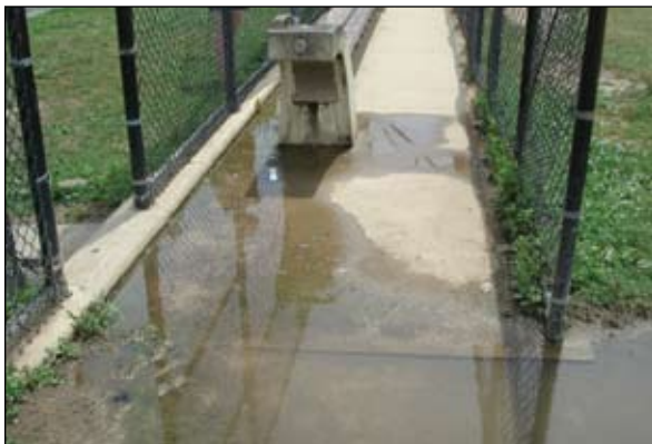
This drinking fountain emits water continuously, creating a large pool of standing water with mold.
