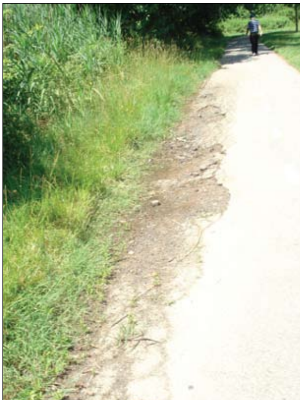
The edges along this path are starting to deteriorate.
