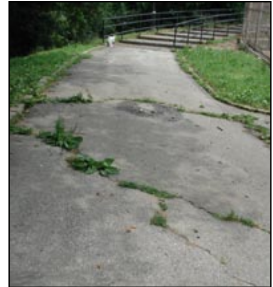
Tremont Park, Bronx, 2006. This pathway, full of trip hazards and weeds, is in need of repair.
